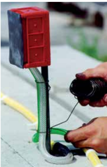
Junction boxes for easy connectivity to hoses
