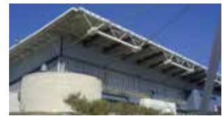
AIS Arena, Canberra (Australia): Sika provided the roofing solution - in service for 34 years already and still performing strongly.
