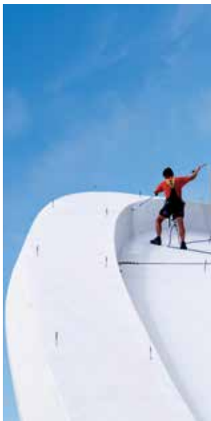
Roofing and reroofing with Sika® Sarnafil® and Sika® RoofPro® MTC membrane systems.
