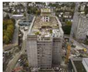
Triemli Hospital, Zurich (Switzerland): Construction featuring recycled and watertight concrete enhanced with Sika® ViscoCrete® admixtures along with other Sika® waterproofing systems.
