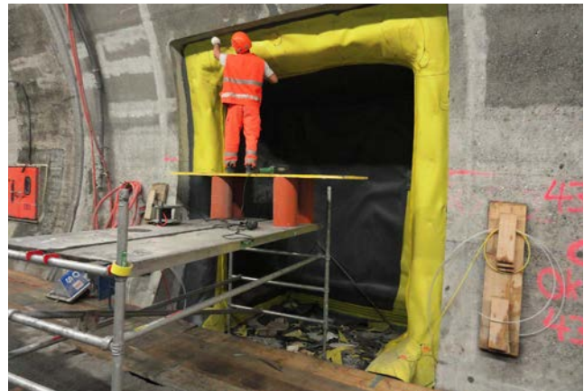
Waterproofing of the excavated tunnel niche using Sikaplan® membrane, directly connected to the existing PVC membrane.
