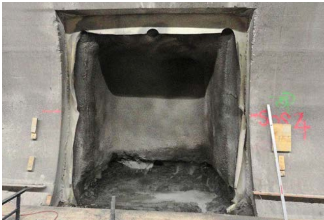
Excavated niche during maintenance works allows accessibility to 44 years old exposed Sika membrane for durability testings.
